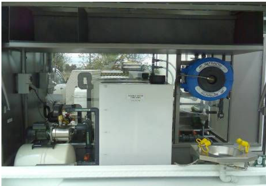
Photo 6—Potable Water System
