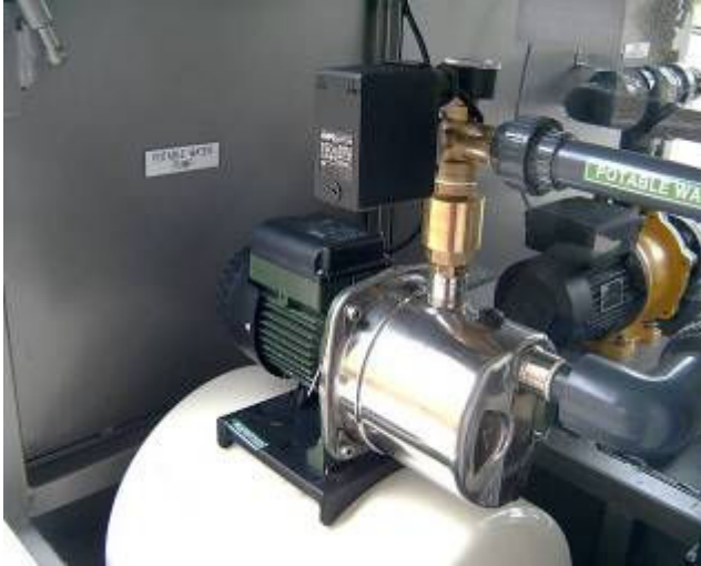
Photo 7 – Potable Water Delivery Pump
