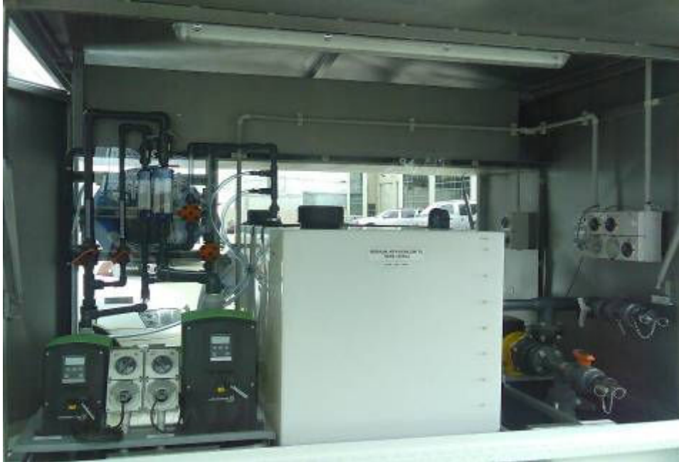
Photo 2 – Sodium Hypochlorite Dosing System.
